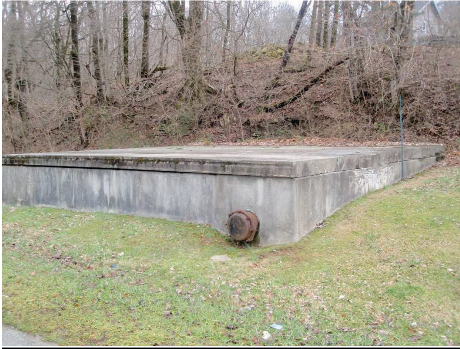
Figure 1. Northeast Pump Station Basin
