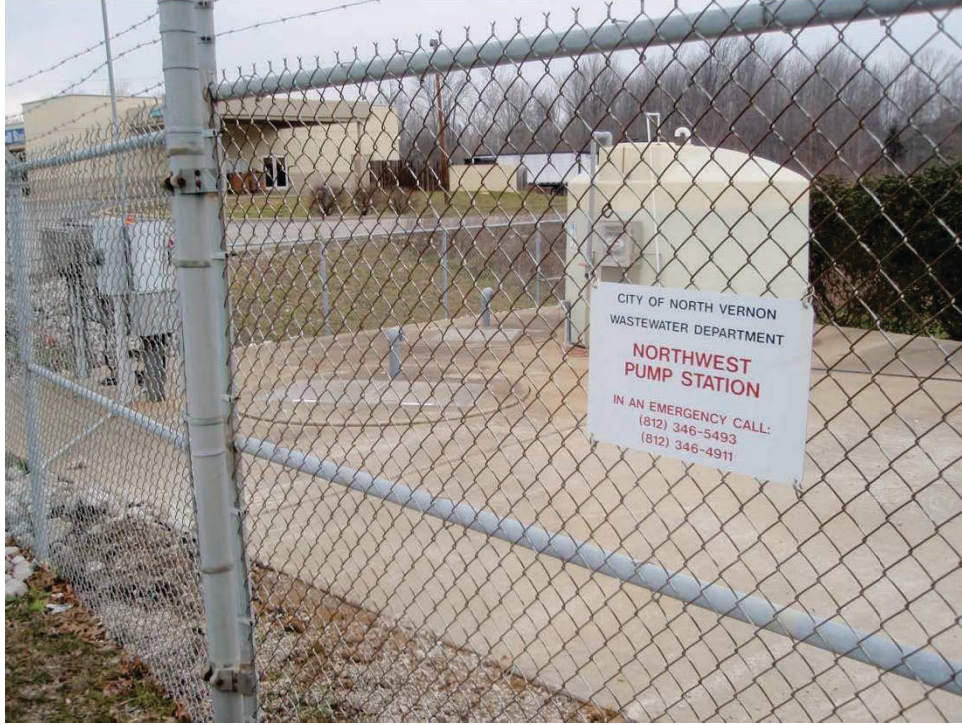
Figure 7. Northwest Pump Station
