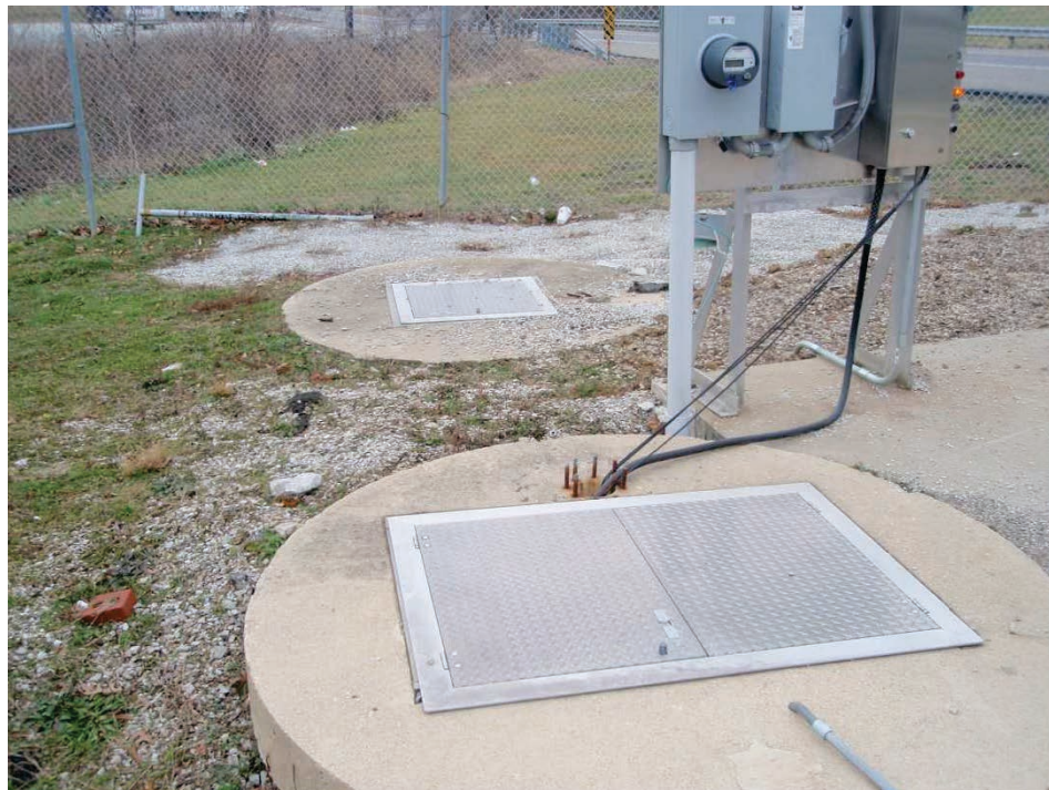
Figure 6. Northwest Pump Station Wet Well and Valve Vault
