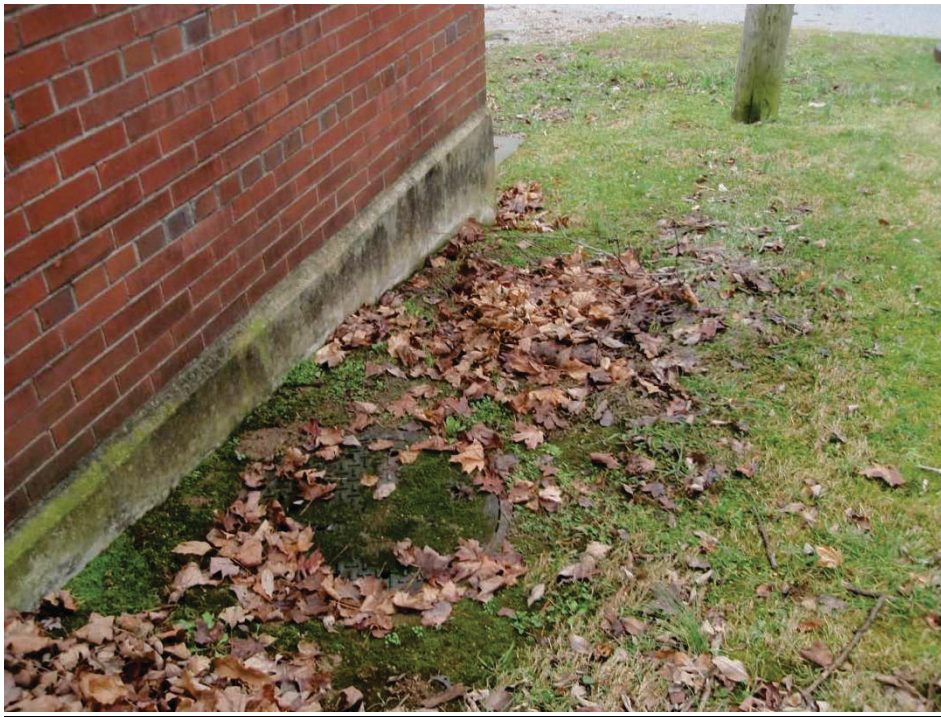
Figure 2. Northeast Pump Station Overflow Point
