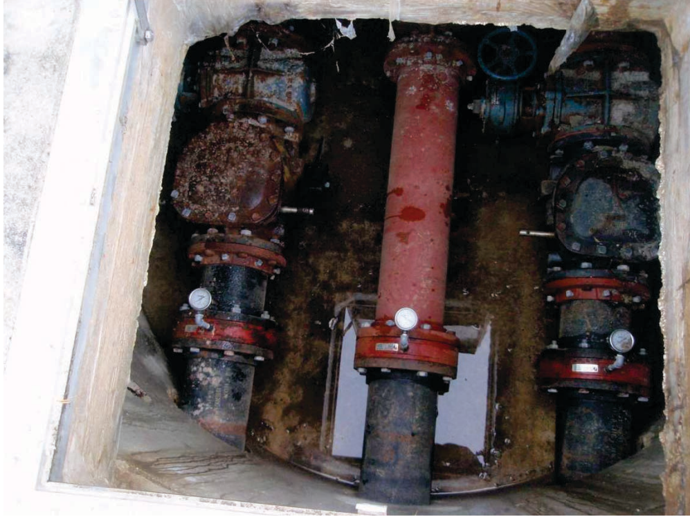
Figure 9. Southwest Pump Station Valve Vault
